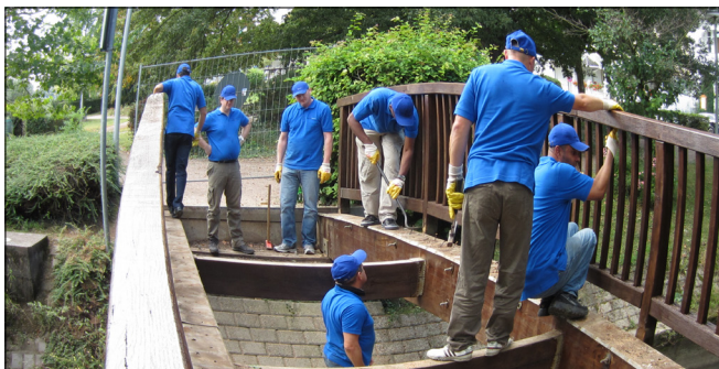
Renovation of a local bus station and two frequently used pedestrian bridges in Walluf, Germany, including a bridge used by the public to safely cross railways
